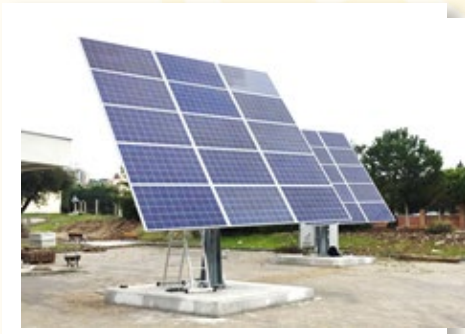
A total of 16kWp photovoltaic power system within Ege University Solar Energy Institute and BESTMER, total energy production: 33.000kWh/year
