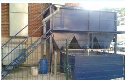
Laundry Wastewater Treatment Plant
