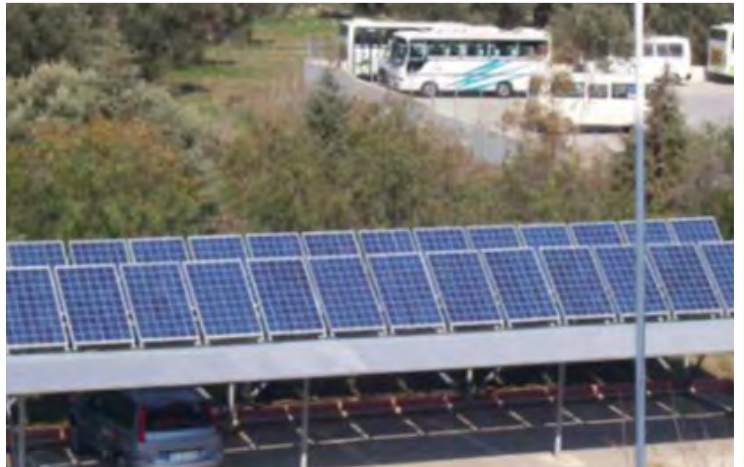
11 AXITEC 150 Wp Photovoltaic Panels, 28 TOTAL TE2000 200 Wp Photovoltaic Panels and 10 Institute Made 120 Wp Photovoltaic Panels (Ege University Solar Energy Institute's Parking Lot).
