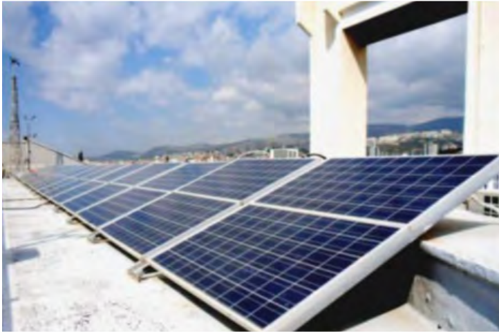
27 TOTAL TE2000 200 Wp Photovoltaic Panel (Ege University Solar Energy Institute's roof)
