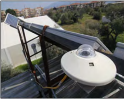
Solar Energy Assisted Heating System.
